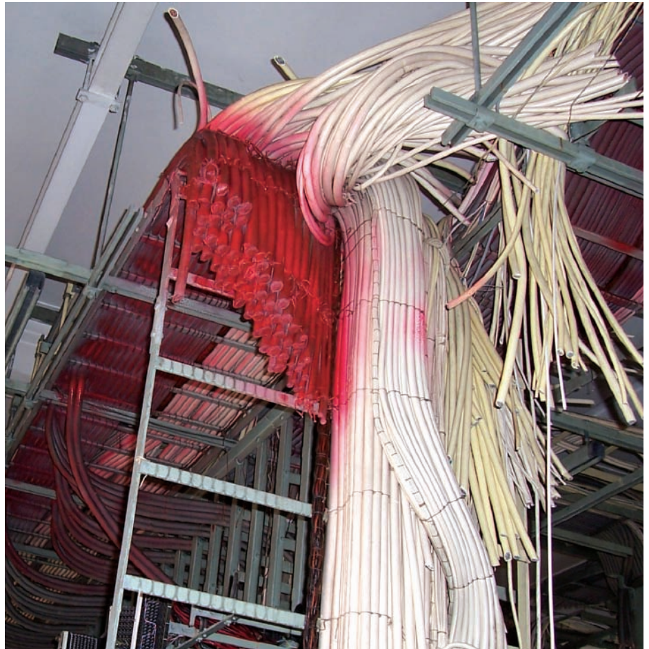
Figure 1. Cotton braided cables in a telephone exchange after treatment with Lead Limiter™ (in red). The Eco Solutions technology penetrates through the cotton braided cable and encapsulates any lead particles into the product, allowing the cables to be safely cut and removed.
